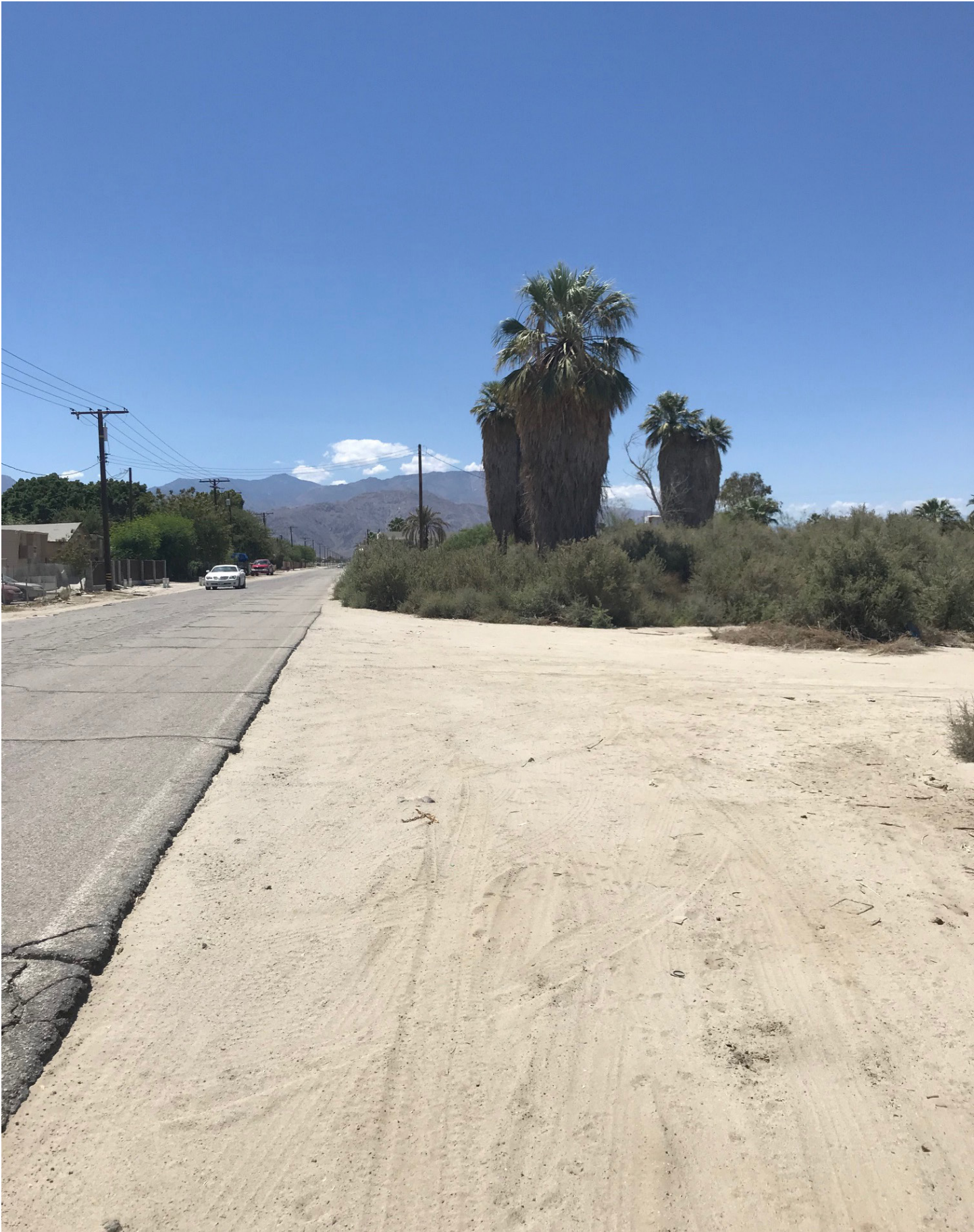
Current condition of Avenue 70 west of the intersection with Pierce Street, identified as a First Priority Corridor
