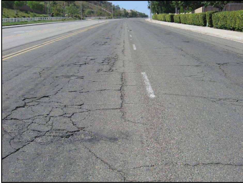
Figure 1E. PCI=30 (Poor Condition)
