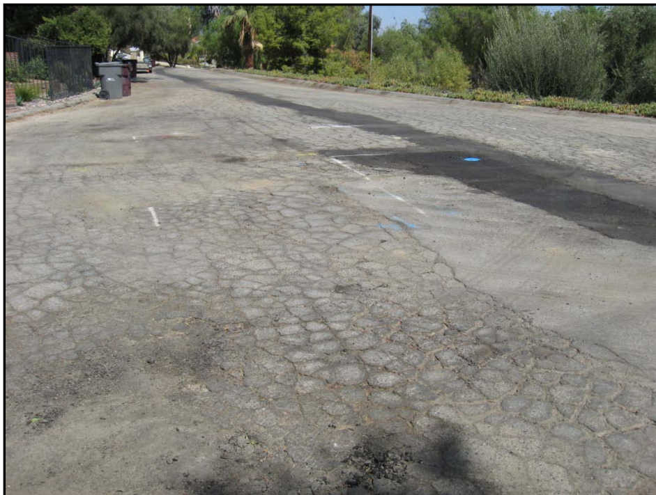
Figure 1F. PCI<10 (Very Poor Condition)
