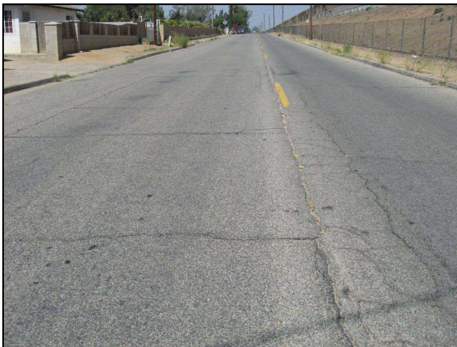
Figure 1D. PCI=56 (At Risk Condition)
