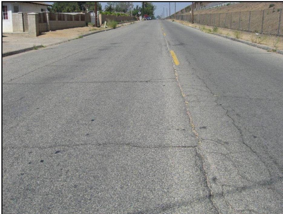
Figure 11D. PCI=56 (At Risk Condition)
