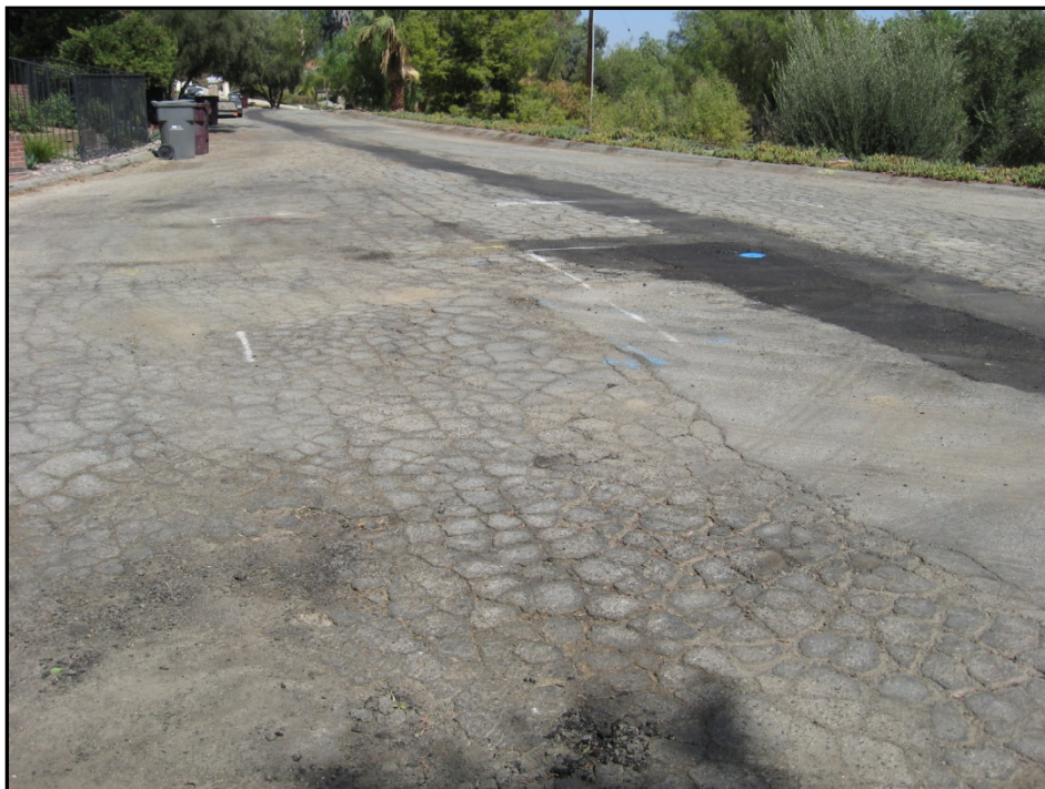
Figure 11F. PCI<10 (Very Poor Condition)
