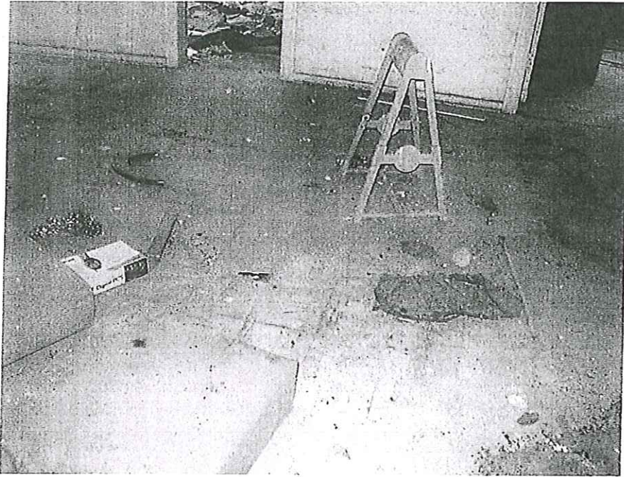
Photograph 1- illustrates the interior of the house living room, the ACM floor tile at 18050 Rice Road, Desert Center.
