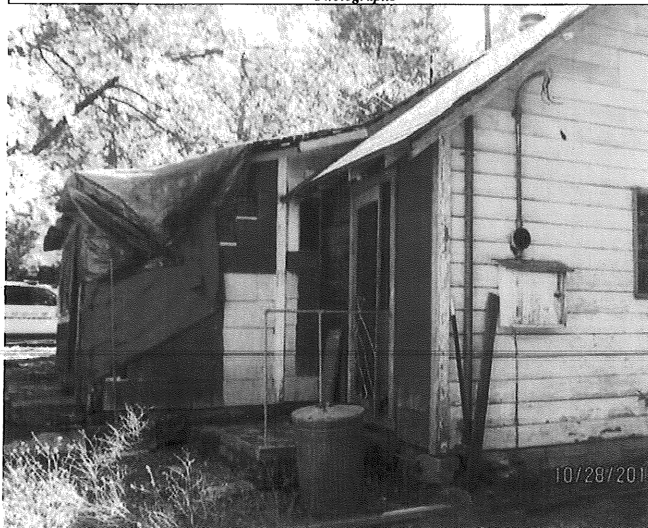
CForrey / Building is still substandard - 10/28/2010
