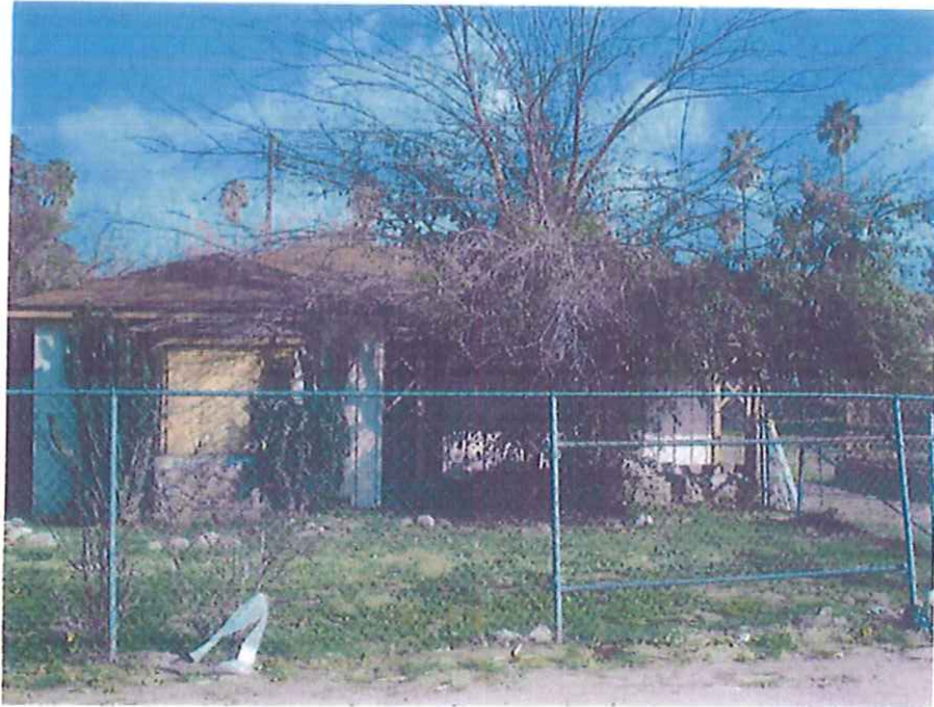
Photograph 1- illustrates the front exterior of house located on the 44174 Florida Ave., Hemet.
