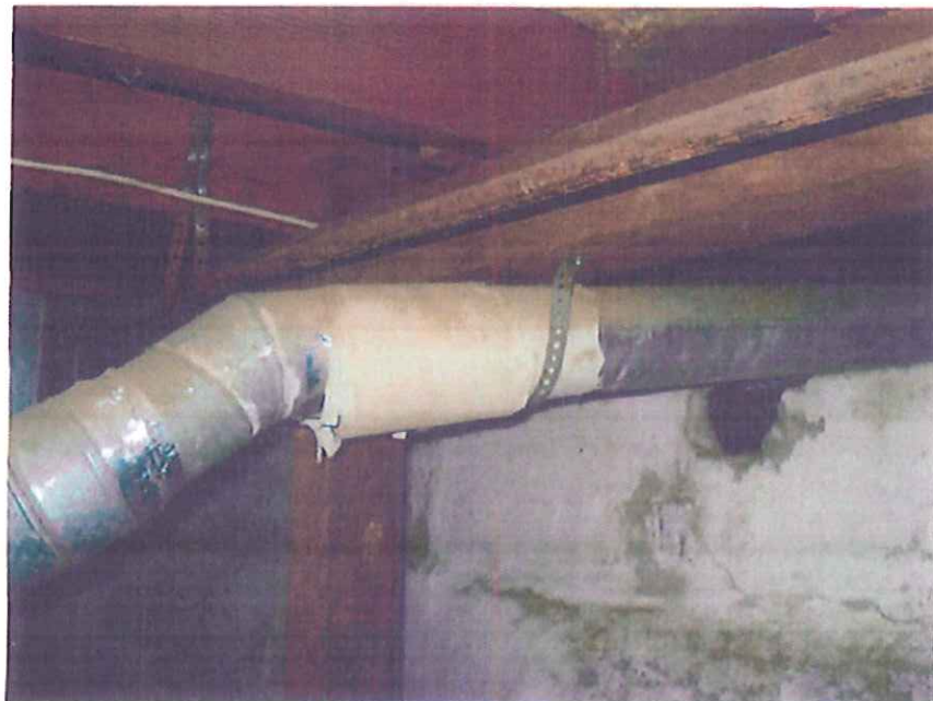
Photograph 2- illustrates the interior of the basement in the main house showing the ACM insulation paper on the metal ducting at 44174 Florida Ave., Hemet.
