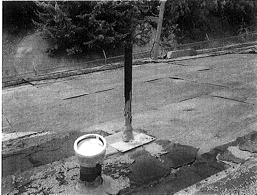
Photograph 2- illustrates exterior roofing mastic penetrations on the roof at 66050 Hwy 74, Mountain Center.
